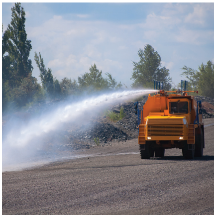
UNPAVED ROADS WILL BE TREATED WITH WATER DURING DRY WEATHER TO SUPPRESS DUST
